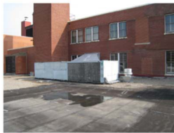
Roof and failed rooftop HVAC unit
