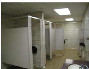
Existing restrooms are worn and lack accessibility
