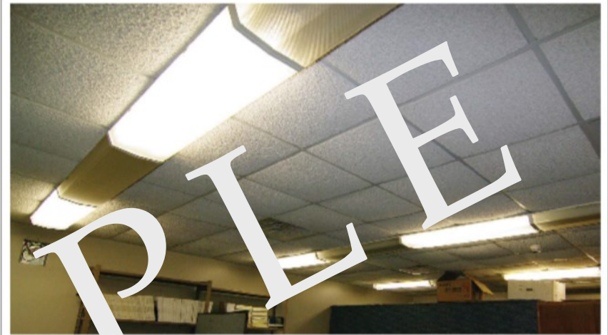
sagging ceiling tile
