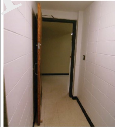
non-ADA compliant door at restrooms
