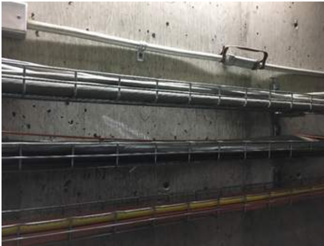
Figure 9: Tunnel cable tray for IT infrastructure
